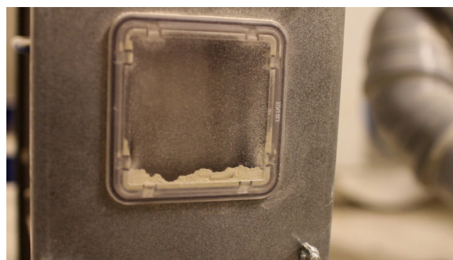
Figure 4. Elevator and dust build up. Overall the entire process produces a lot of fine dust. Photograph: Casimir Schauman
